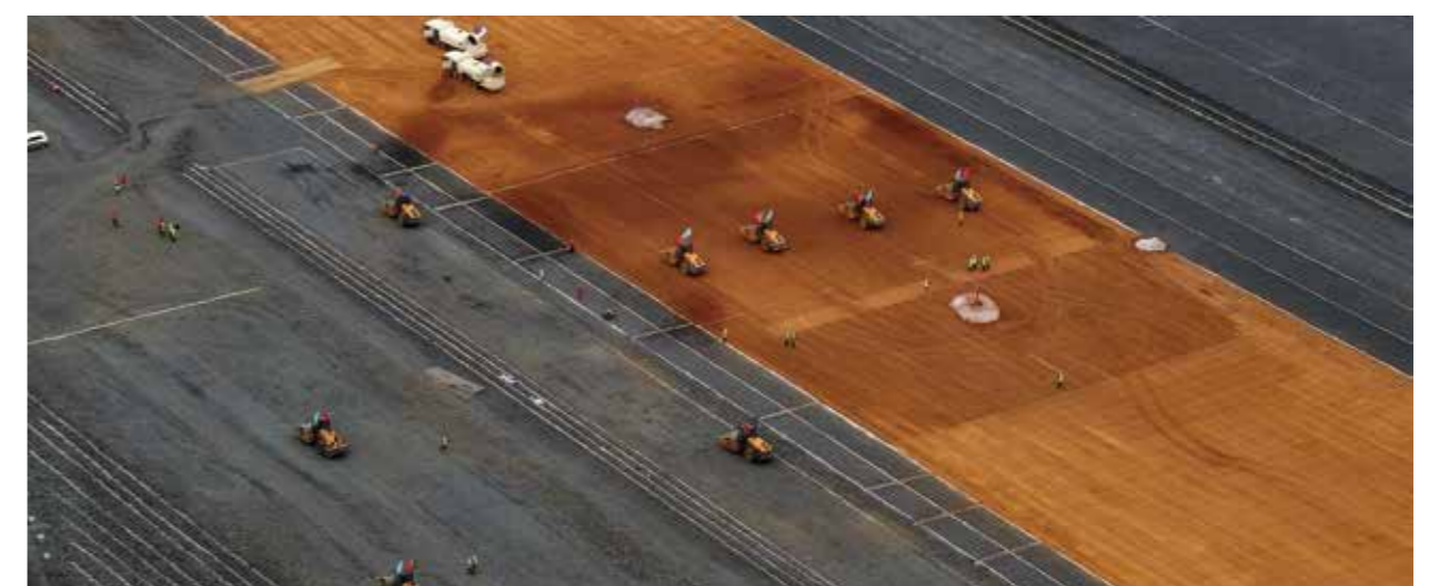
Construction site of the core-wall for earth-rockfill dam at Yalong River Lianghekou Hydropower Station
