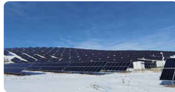
24MWp PV power project of Guyuan Guanghui New Energy Power Generation Co.
