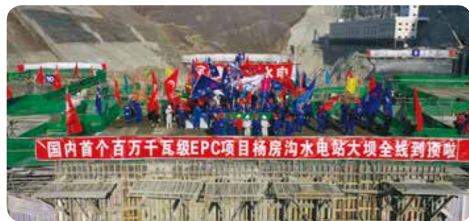
Concrete pouring completed in construction of Yangfanggou hydropower station along the Yalong River
